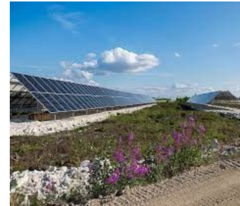
Solar panels in Old Crow.
